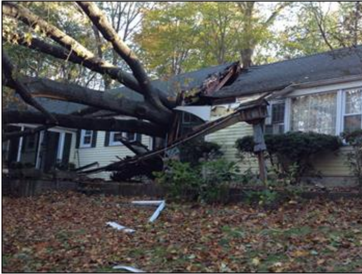
Figure 1 Property Damage from Fallen Tree
